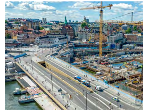
Slussen, Stockholm, Sweden A 400-year-old landmark, remade for a new era. Page 59
