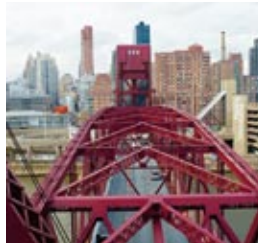
Roosevelt Island, located in New York City's East River, is reachable by car only via a lift span bridge constructed in 1955. The bridge – linking the borough of Queens with the island – has now been totally refurbished by Skanska, which received the assignment on the basis of its bridge expertise, not its price. The project was completed two months ahead of schedule.
