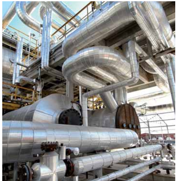
Petrobras Sulfur Recovery Unit, São Paulo, Brazil.
