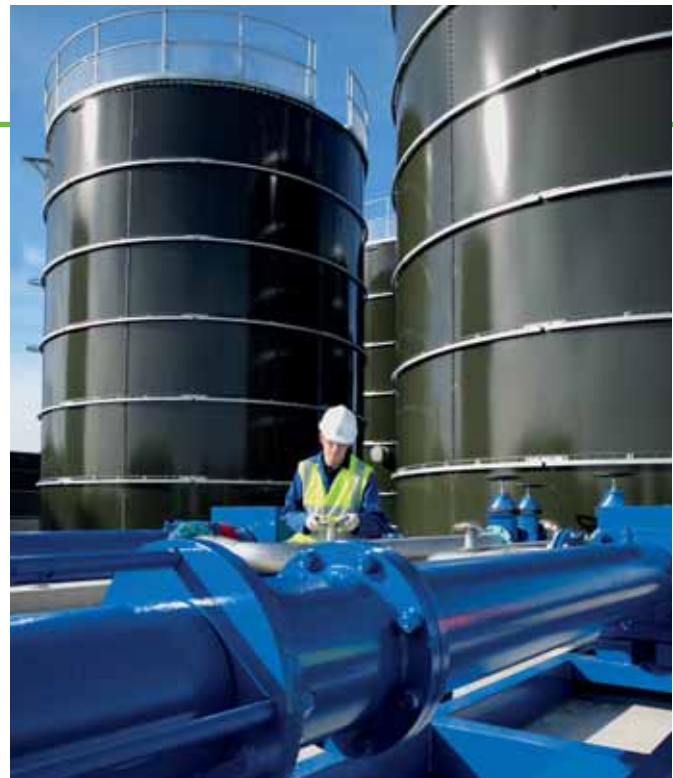
Water treatment facilities for Anglian Water, U.K.
