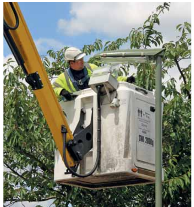
The newly installed street lighting network in Surrey, U.K. is energy-efficient thanks to a central control system.
