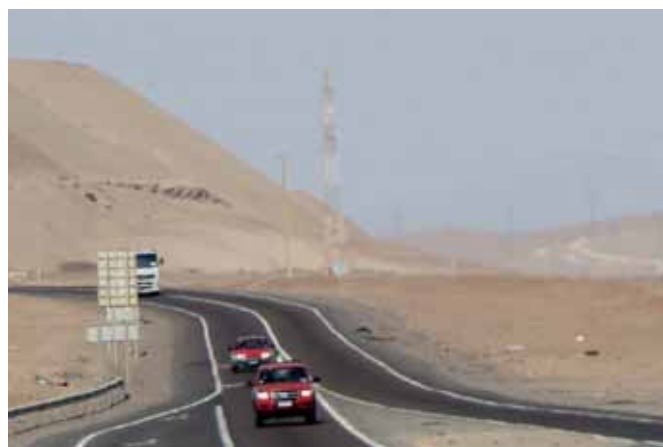
Construction of a new 120 km (75 mi.) long section of highway in Antofagasta, Chile.
