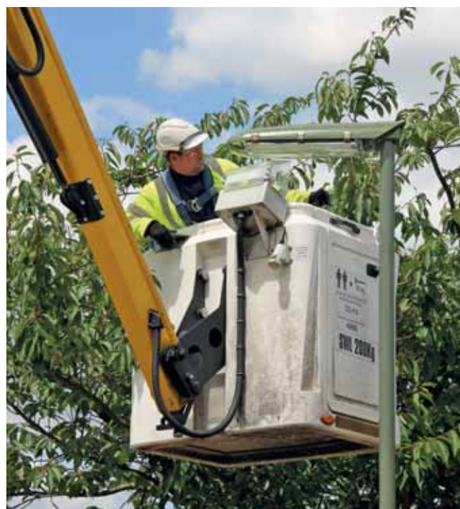
The newly installed street lighting network in Surrey, U.K. is energy-efficient thanks to a central control system.
