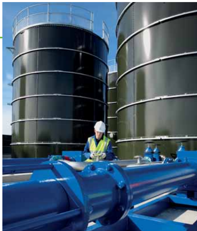
Water treatment facilities for Anglian Water, U.K.
