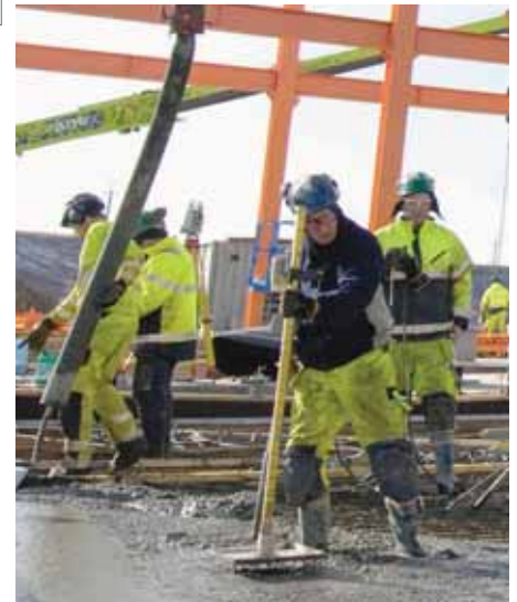
Up to 1,500 people are working on the construction of New Karolinska Solna in Stockholm, Sweden.
