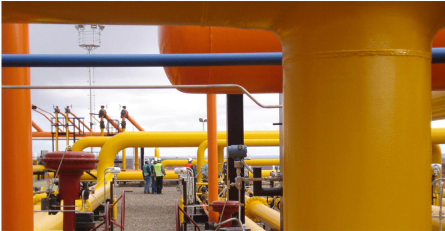
"El Casquete" primary separation unit and compression plant, Neuquén, Argentina
