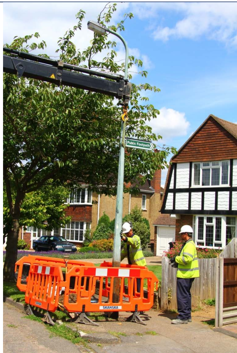
Surrey street lighting, U.K.
