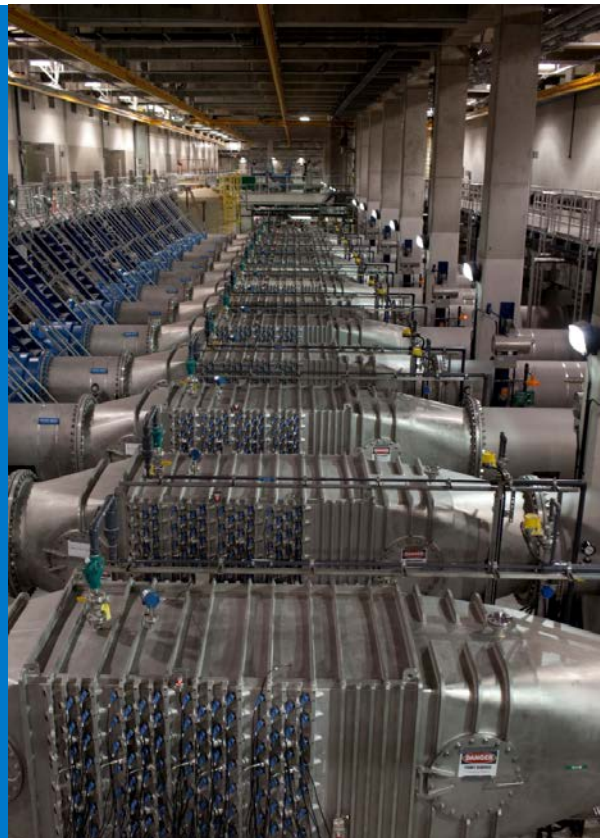
Catskill/Delaware UV Water Treatment, NYC, USA
