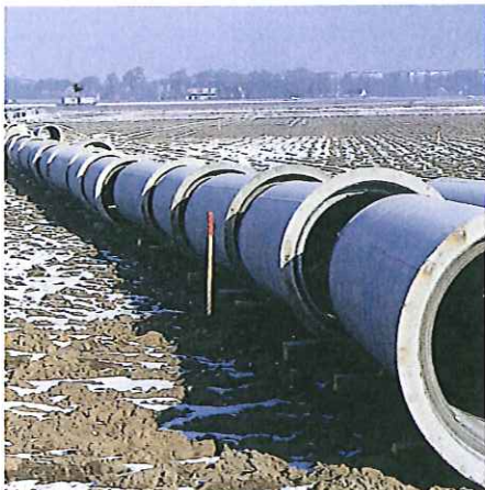
Piping for a 24 km (15 mi) untreated water pipeline – part of the Lake Bolmen fresh water supply system.
