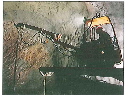
Underground reinforcement is one of Stabilator's specialties. At the Hylte power plant, subterranean tunnels were reinforced with shotcreting and grouting.
