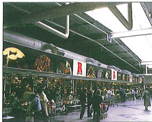
IV was responsible for supplying the ventilation system at the Mobilia department store in Malmö.
