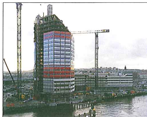
Engdahl Stålteknik delivered a complete steel frame and a glass and aluminum façade for the Lilla Bommen project in Gothenburg.
