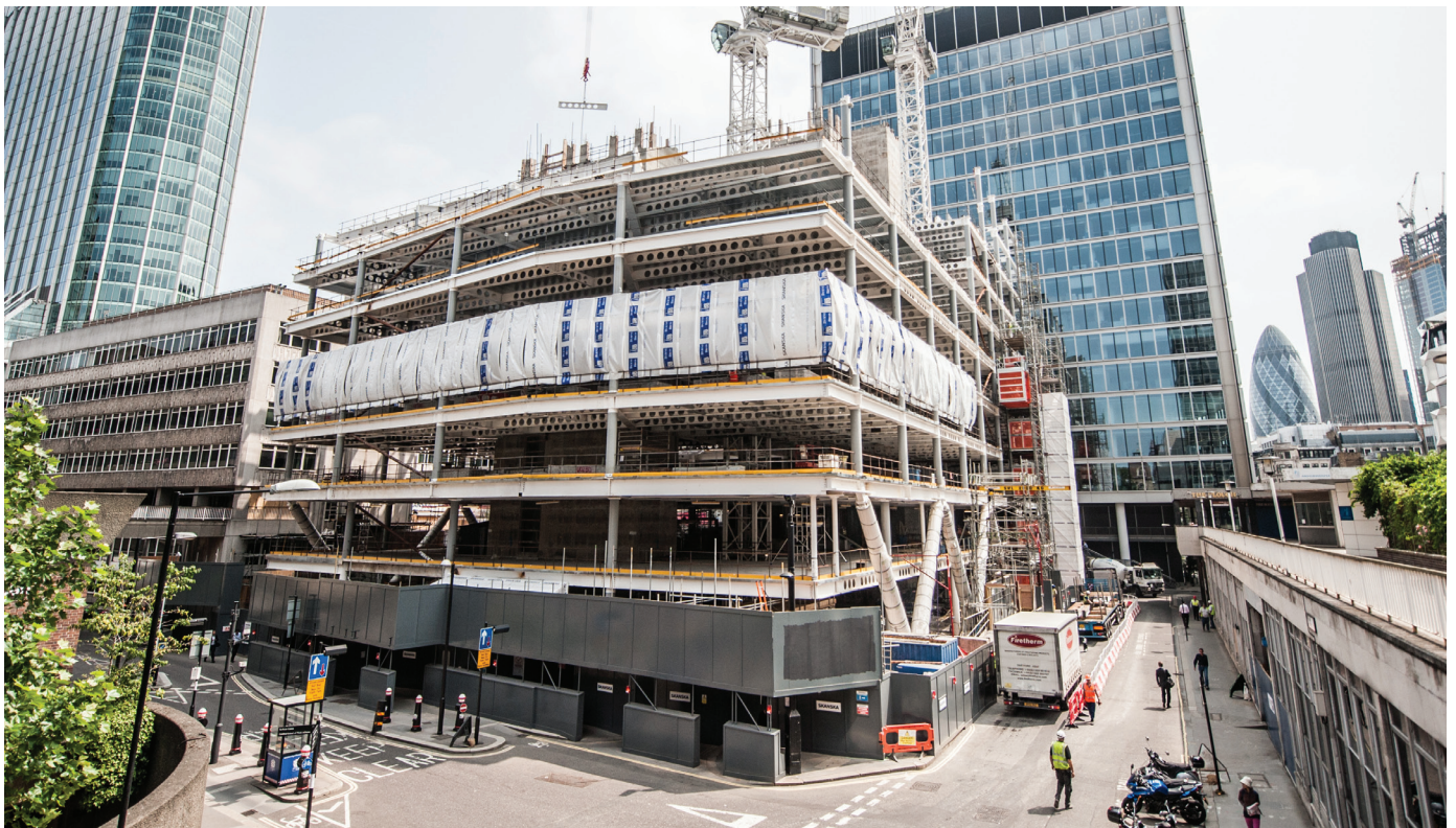
Moorgate Exchange, London, UK.
