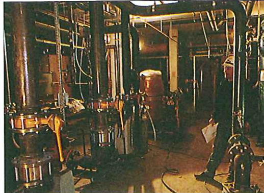
Extensive plumbing and heating installation work for Visby General Hospital was one of Skanska Installation's major 1991 orders.
