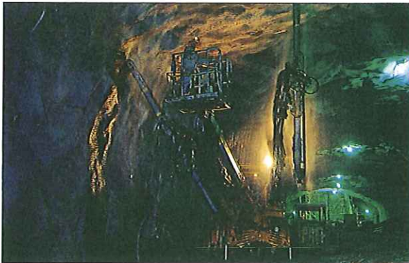
Skanska has long experience of Stockholm subway system expansion. Several Skanska units are working together on the current extension of the southeastern line to Skarpnäck.
