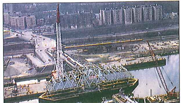
Portions of the original bridge span were re-used in this remodeled swing bridge over the Harlem River, produced by Karl Koch.
