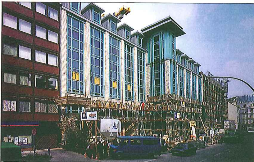
The ongoing ABC-Strasse residential and office project in Hamburg, Germany, will be ready for occupancy in 1992. Skanska Baugesellschaft is the project and construction manager.
