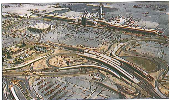
Slattery Associates is building a new traffic interchange, with 9 km (5.5 mi) of highway and 2.5 km (1.5 mi) of elevated road, at New York's John F. Kennedy International Airport.
