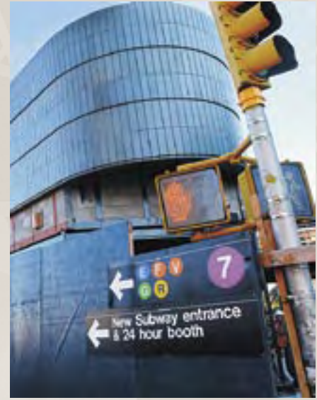
The Roosevelt Avenue/74th Street subway station is the site of one of numerous major infrastructure projects underway in New York City, where Skanska is the largest construction company. The station is undergoing a large-scale reconfiguration and renovation, costing about SEK 630 M.
