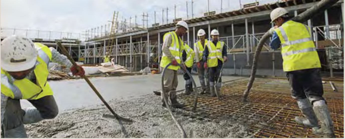
In Derby, construction is underway on a new hospital that will be operated as a public-private partnership. The British term for such projects is Private Finance Initiative (PFI). Skanska BOT holds half the ownership consortium, and Skanska UK has the full design-build contract for the hospital, worth GBP 333 M. The first half of the 155,000 sq. m (1.68 million sq. ft.) project will be completed in 2006.
