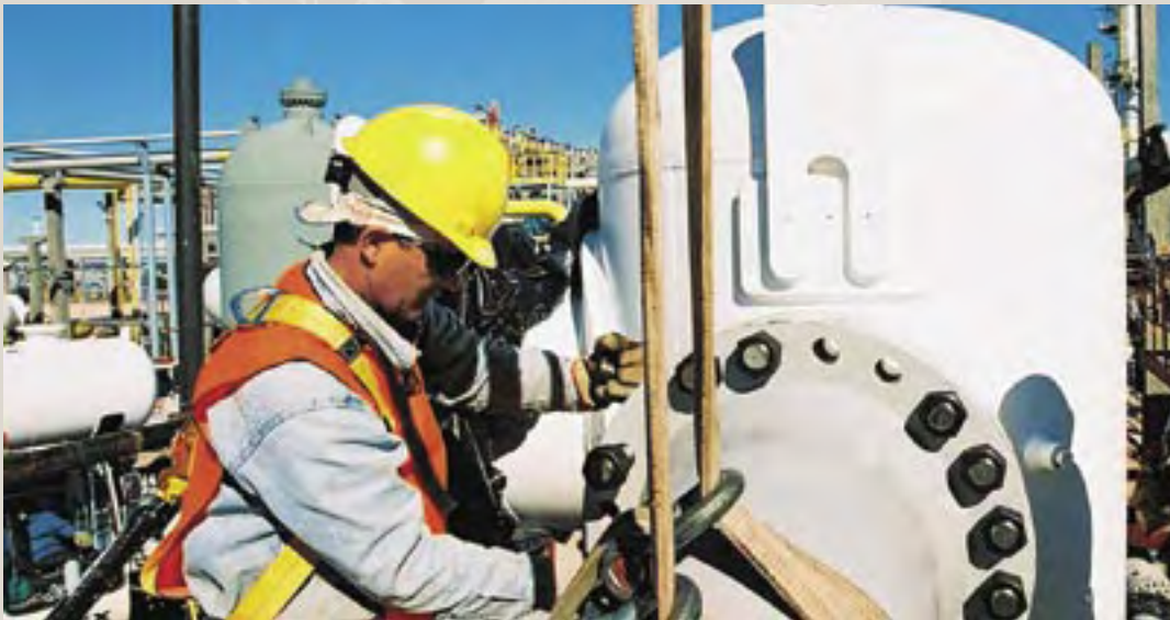
International energy companies are major Skanska customers in Latin America. During 2004, the company completed an expansion of the Loma de la Lata gas production plant in Neuquen, Argentina.
