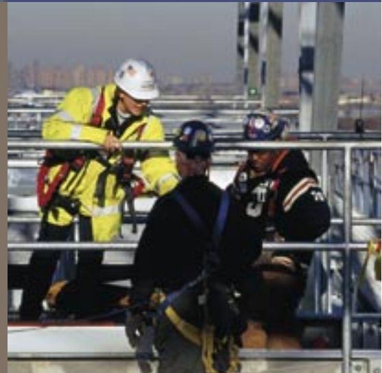
Charles M. Poletti Generating Station, New York City, U.S.A.
